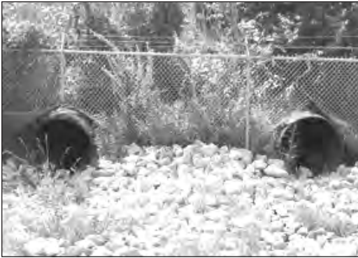
FIGURE 1. Culverts through a fence line can create large passageways for wildlife at airports. (Photo by J. E. Kubel)
