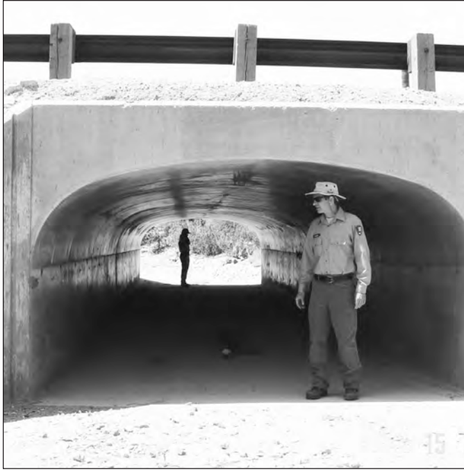
Figure 1. Saguaro National Park and Pima County, Arizona, collaborated to design and construct a wildlife-friendly culvert on Sandario Road adjacent to the park. (Photo courtesy National Park Service)
